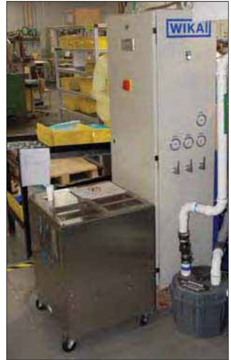
Chillers Reduced Water Consumption at WIKA
