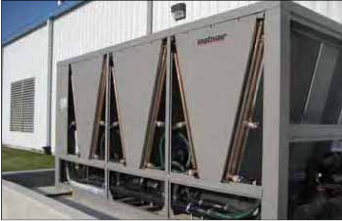
Hydraulic Hose Glycol Connections to the Integrated Free-Cooling Coils
