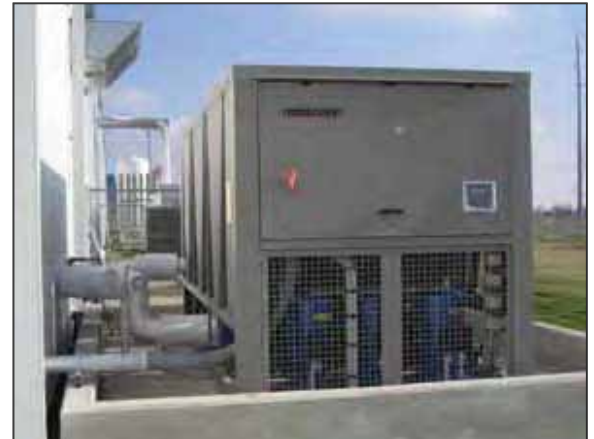
Motivair Free-Cooling Chiller Installed at a Steel Tube Mill
